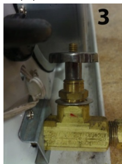
fusible link valve
